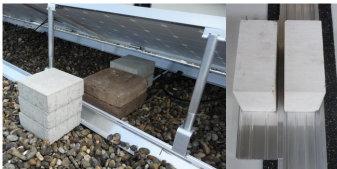
Figure 27 Ballast distribution: on base troughs (left) or via the ballast trough (right)
